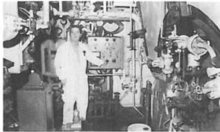
Crewman monitors controls for one of the four boilers in the engine room of the Princess Marguerite.
